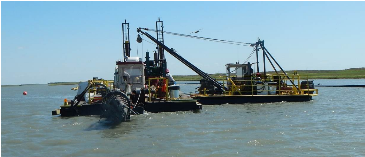
Figure 1. The hydraulic dredge mobilized to the start of the Cedar Bayou dredging.
